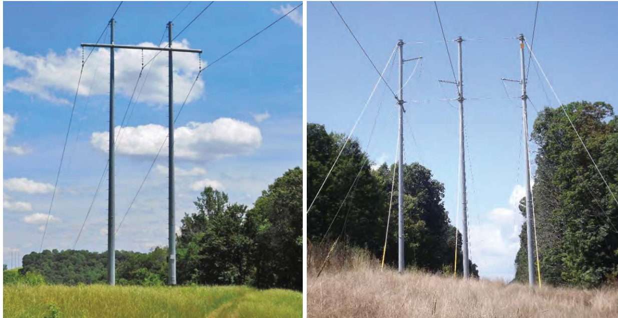
Figure 2. Typical Transmission Line Structures H-frame (left) and Three-Pole Dead End (right)
